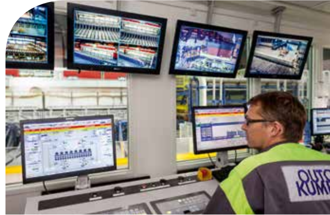
The thermal treatment line is equipped with our X-Pact® electrics and automation.
